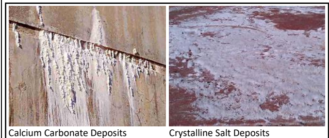
Calcium Carbonate Deposits
